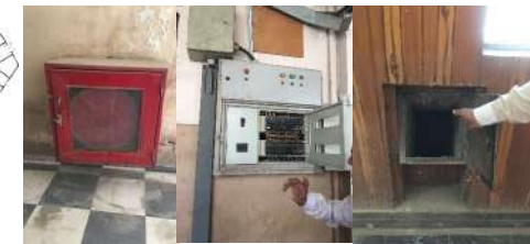
(Fig.66) Existing firefighting, electrical and garbage system units. Source: Author
