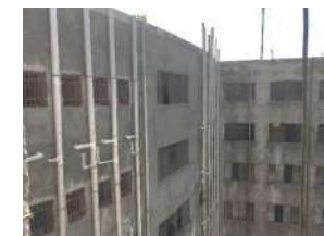
(Fig.60) - Exposed public toilets pipes in the court. Source: Author, 2022
