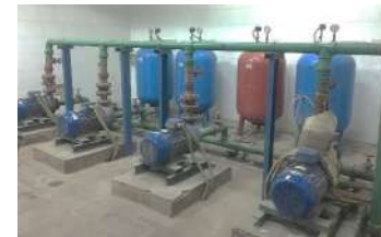
(Fig.61) - Al-Tahrir building existing pumps room. Source: Author, 2022
