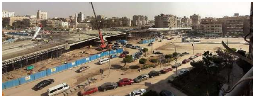
Figure 35: El-Hegaz square before and during the construction of the flyover – Source: Facebook page (Ana min Masr Alqadida , 2019)
