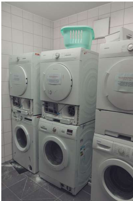
Figure (4.30) The Washing Machines and Dryers in the Laundry Room Source: Author
