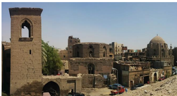
Figure 5 Visible groundwater seepage issues beneath two historic monuments, al-'Ashraf Khalil Shrine (the dome on the right) and FātimaKhātūn shrine, Source: (Tadamun, 2019; al-Ibrashy, Ibrahim and Samir, 2022).
