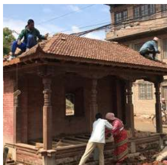
(fig. 31)—Community members helping in the construction of destroyed Pati Source: mohr-stiftung.de
