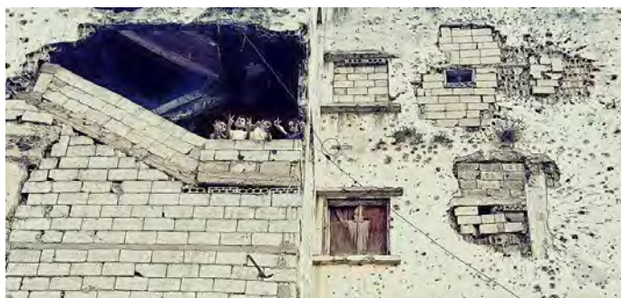
(fig. 62)—Abandoned Building in Badaro where a refugee family is living inside of it. Source: Warde (2016)
