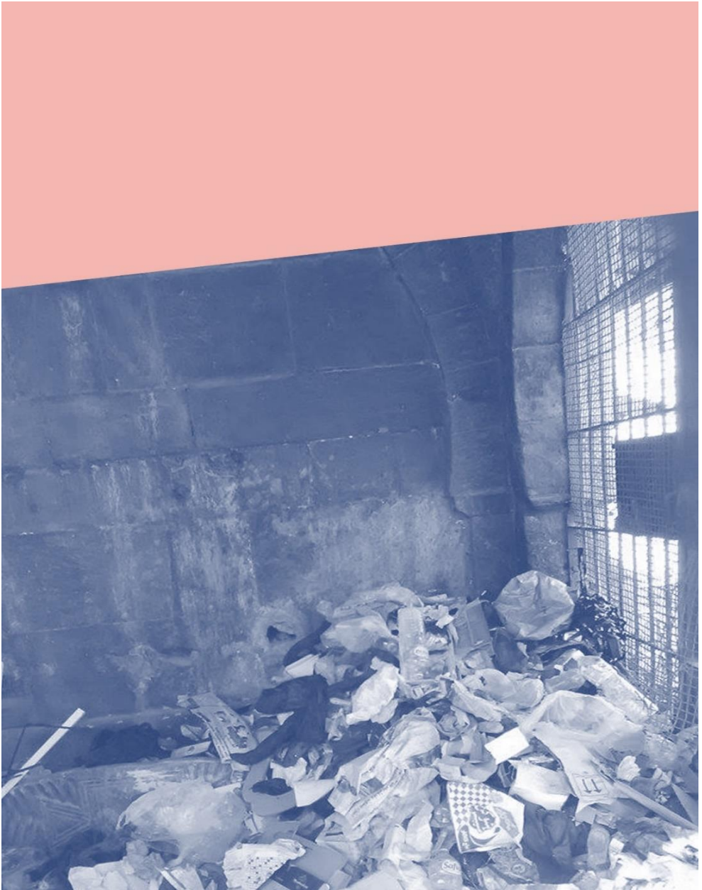
Figure 39- State of the fountain as of June 2016. Photo: Boubaker Ben Fraj, 2016
