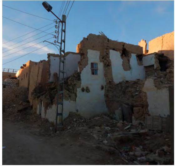
Fig.30: Deteriorated vernacular house, source: author,2016.
