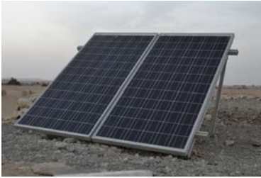
Figure 7.17: Domestic PV system on the roof top of a house
