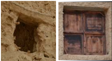
Figure 6.09: Left: A window opening supported by palm tree trunk from the upper side
