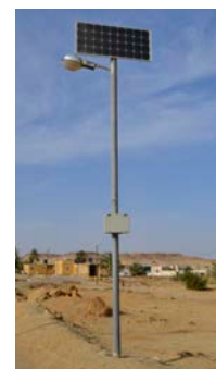
Figure 5.19: PV street lamp
