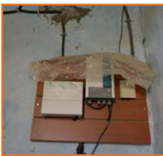
Figure 6.61: PV internal control panel
