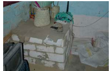
Figure 5.23: Indoor built-in corner holding the batteries inside
