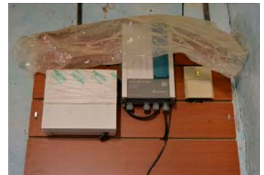
Figure 5.22: The indoor control panel
