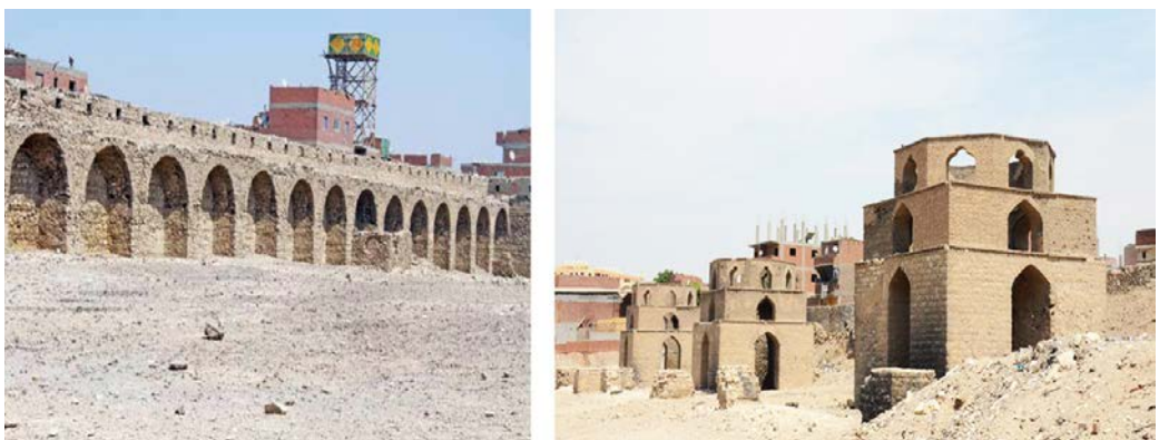
Figure 4-6: Deterioration conditions of monuments in Ezbet Khyrallah. Establ Antar (Left), and Sabaa Banat (Right) (Source: Tadamun, 2013).
